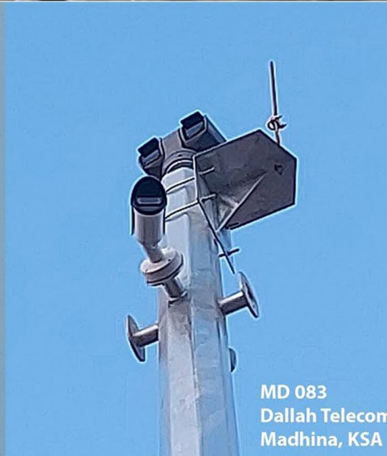
MD 080 Dallah Telecom Madhina, KSA
